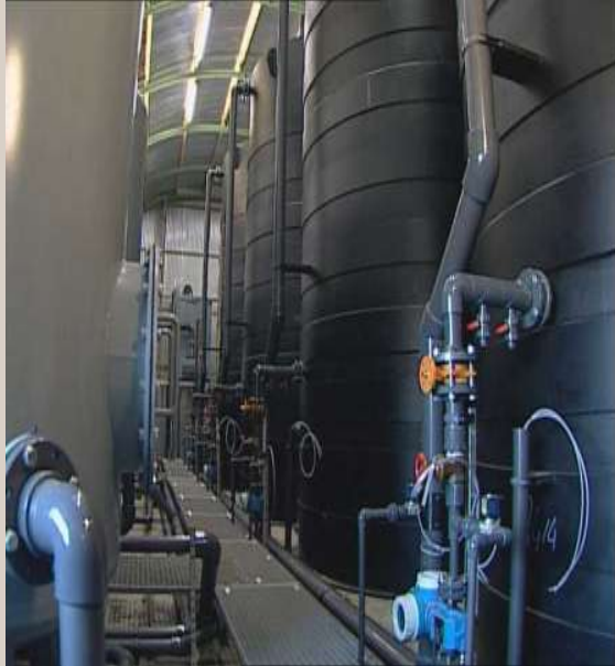
Fixed system, 100 m 3 reactor
